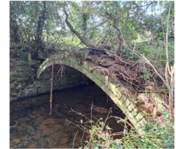
4 The remains of a historic arched bridge, upstream of the railway bridge.
