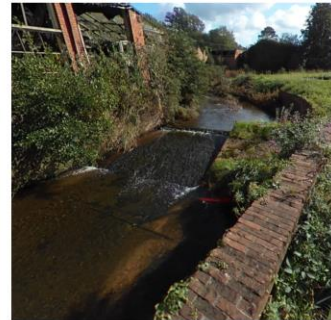
2 Small weir on the at the Tonedale Mill site. River banks in this section are brick banked. The condition of these was not assessed.
