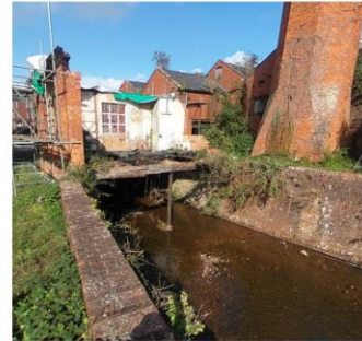
2 Historic culverted sections are structurally in very poor condition with visible sagging of the soffit of the structures.
